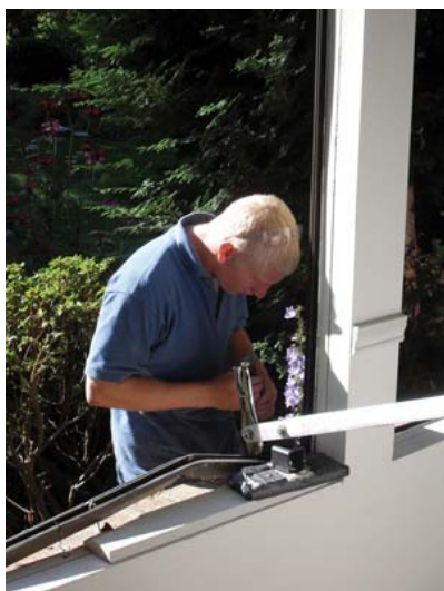
All of Penguin's installations are completed according to InstallationMasters guidelines and employees are encouraged to make time for the details.
